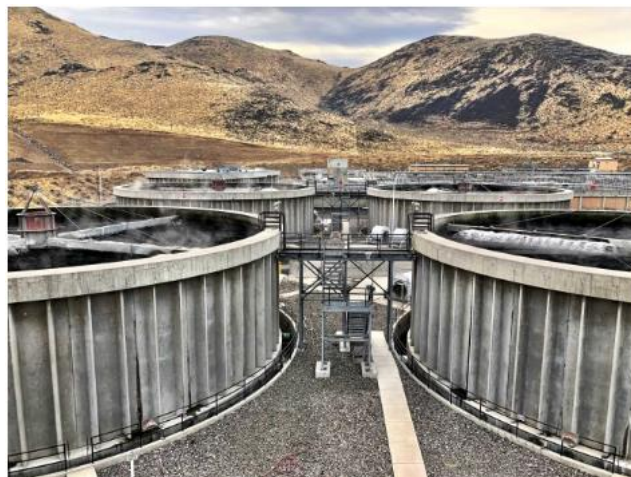
Figure 11 TMWRF facility, via TMWRF website
