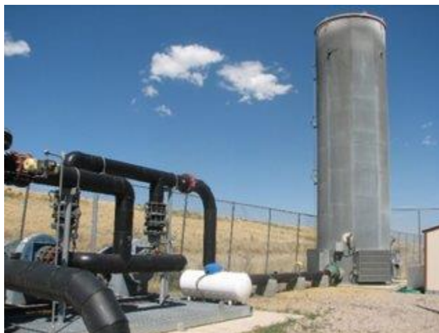
Figure 9 Example of an enclosed LFG flare, from EPA website
